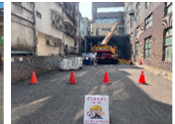
No Entry to Construction Zone
