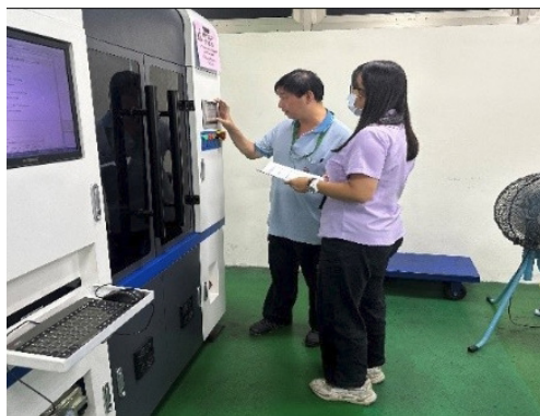
After Improvement: Safety Interlock Devices Installed on All Safety Doors
